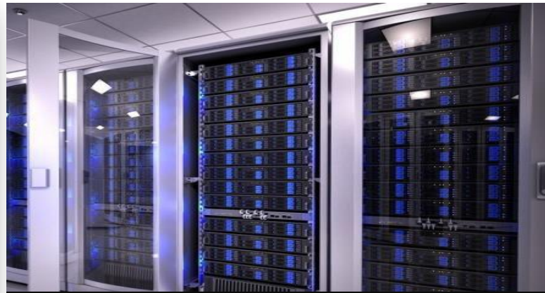
Enterprise power & telecom
