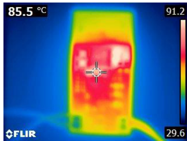
Figure 9. Thermal Image at 15.0 A Load
